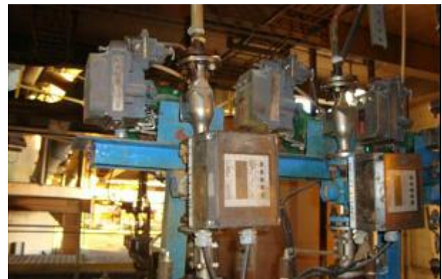
Figure 4: individual flowmeters in each line of the dosing system with centrifugal pumps
