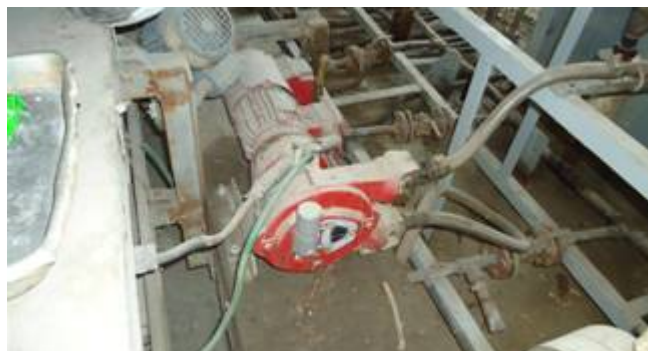
Figure 5: Peristaltic pump SPX10 installed for the tests
