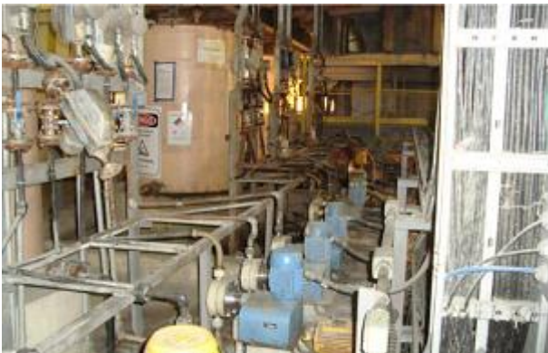
Figure 1: Dosing system with diaphragm pumps
