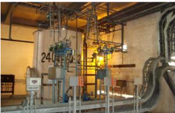
Figure 3: Dosing system with centrifugal pumps
