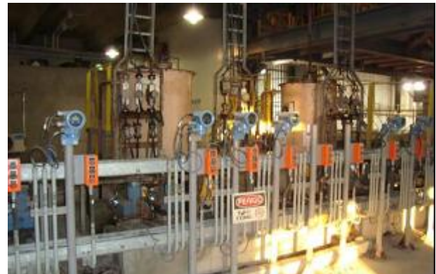
Figure 2: individual flowmeters in each line of the dosing system with diaphragm pumps
