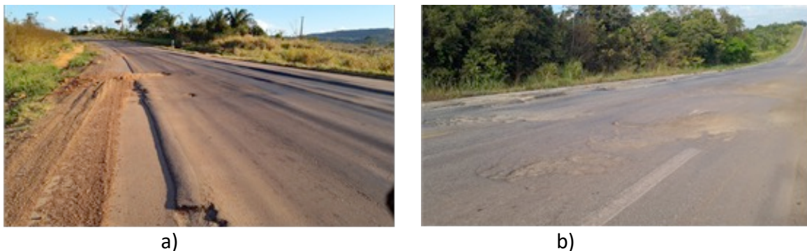
Figure 8: Pavement conditions in Pará federal roads - a) BR - 163; b) BR - 222.
