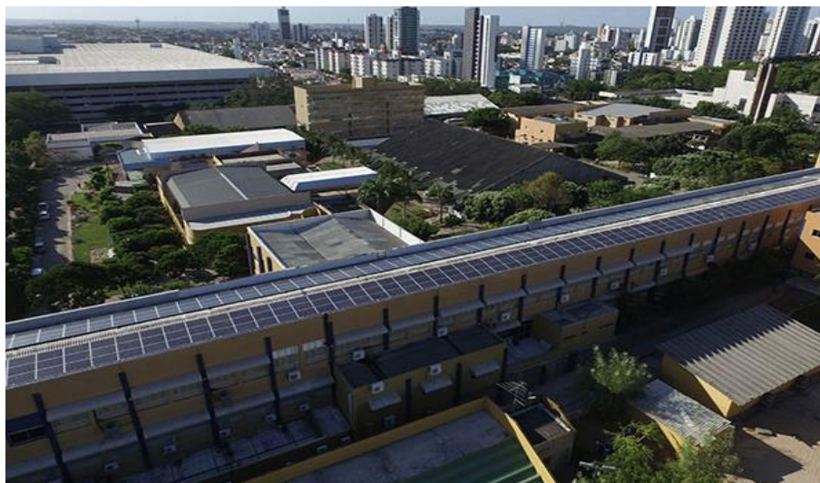
Figura A9: UFV IFRN NATAL-CENTRAL: 480 painéis de 235 Wp + 345 painéis de 245 Wp = 197,3 kWp.
